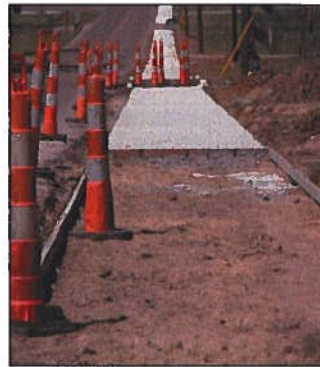
Leader photo by NANCY BERGERON Construction is underway on the sidewalk connector that will eventually run from near I. A. Lewis School to Green Clinic. So far, 1,300 feet have been completed.
